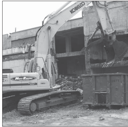
photo—Jon-Michael Higgins, courtesy Level 2 Development. Shown here during the well-attended “groundbreaking” event on July 25th is a clear sign that the old Petrovitch building demolition is moving along, to be replaced by the ambitious View 14 development.
